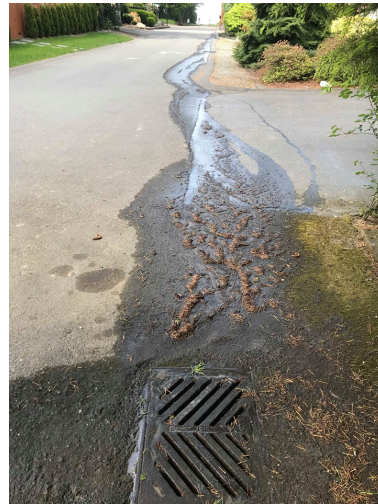
Photo 9 (looking N): Type 1 Catch Basin (#5). 12" concrete inlet according to GIS, but appears to be 6".
