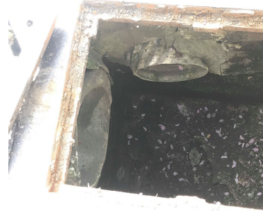
Photo 2 (looking into CB #1): 12" concrete inlet from the south and 8" corrugated inlet from the
