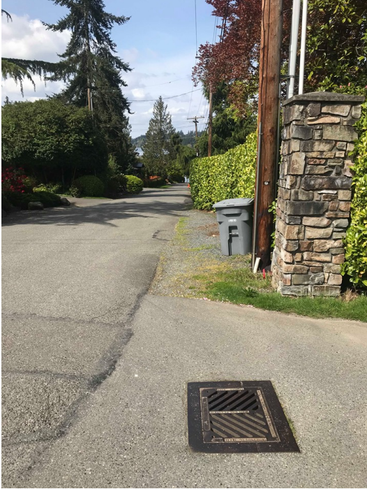
Photo 1 (looking N): Type 1 Catch basin (#1). 12" concrete inlet from the south and 8" corrugated inlet from the southwest. This CB will be receiving runoff from the project development.
